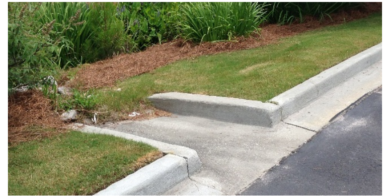
Figure 4.08.2. Concrete Curb with Drainage Opening
